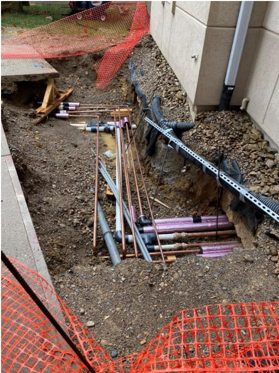
Norse Hall, New Underground Piping (Copper Pipe Replaces Blue Max Piping), July 2020
