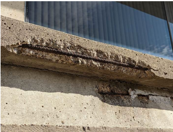
Spalled concrete slab edge/exposed rebar
