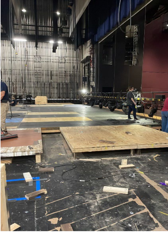
Corbett Stage False Floor (installed by SOTA to create a flat surface for safety) being Dismantled
