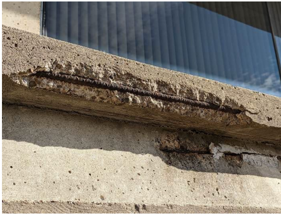
Spalled concrete slab edge/exposed rebar
