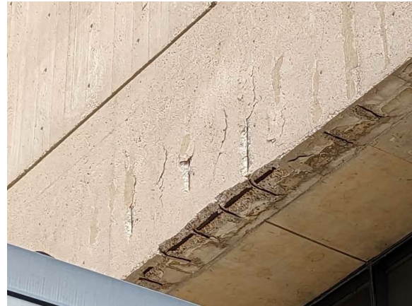
Concrete vertical surface spalling
