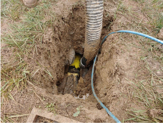
Steel and Plastic Pipe Juncture near Norse Commons
