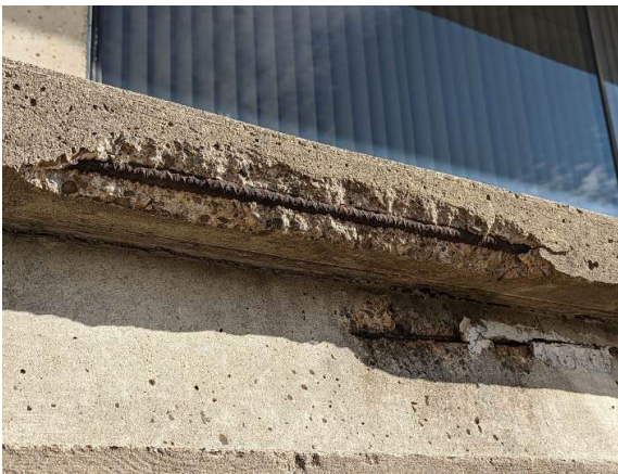
Spalled concrete slab edge/exposed rebar
