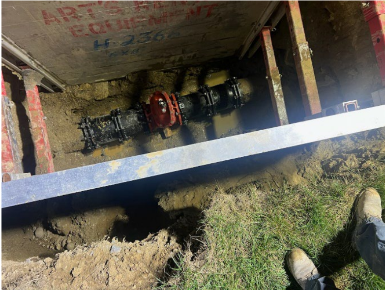
Replacement Water Valve
