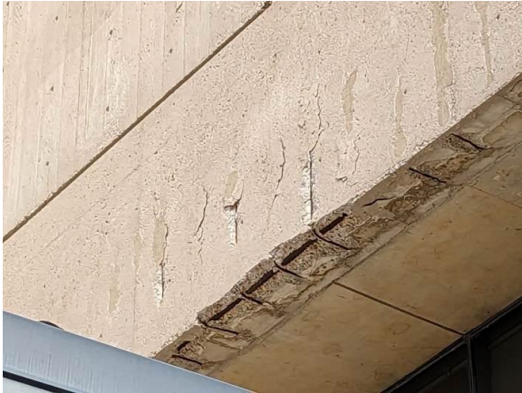
Concrete vertical surface spalling
