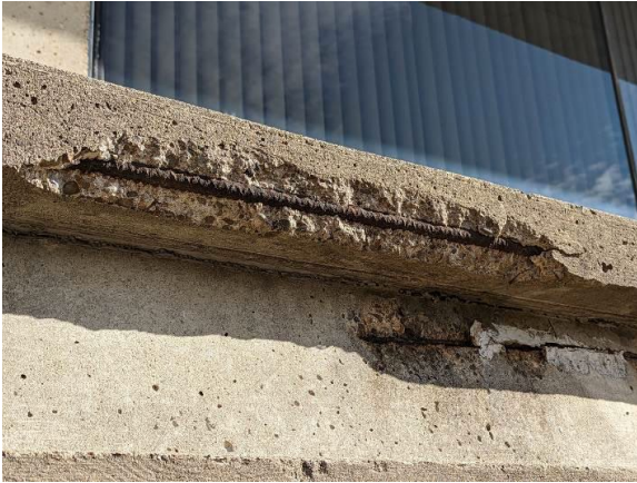
Spalled concrete slab edge/exposed rebar
