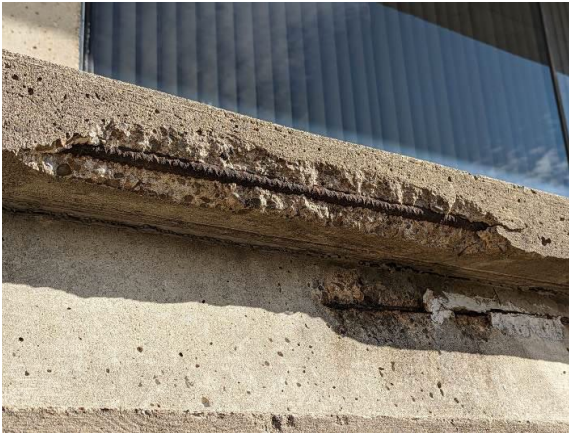
Spalled concrete slab edge/exposed rebar
