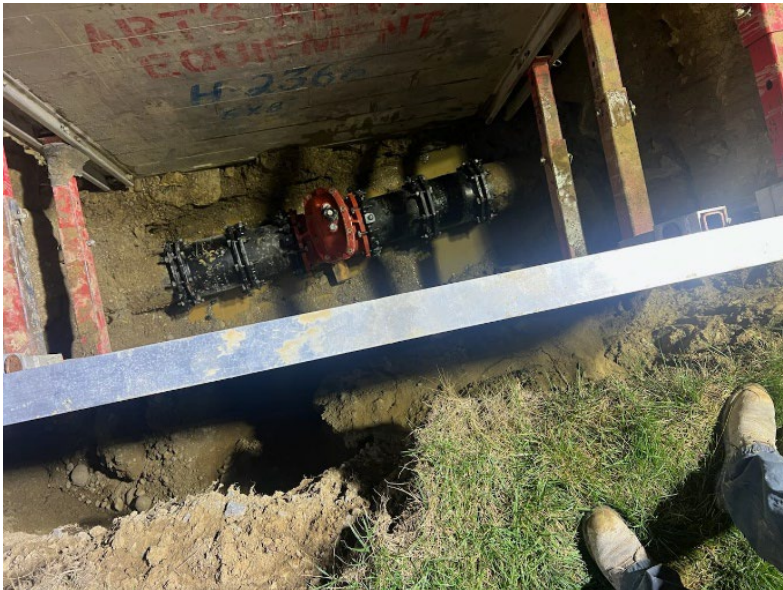
Replacement Water Valve
