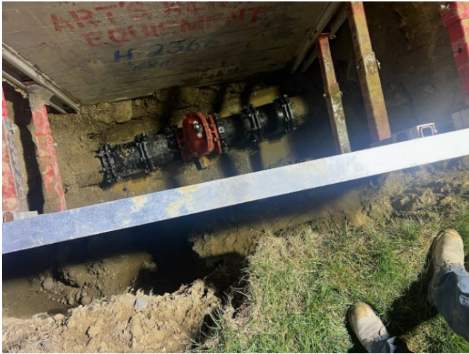
Replacement Water Valve
